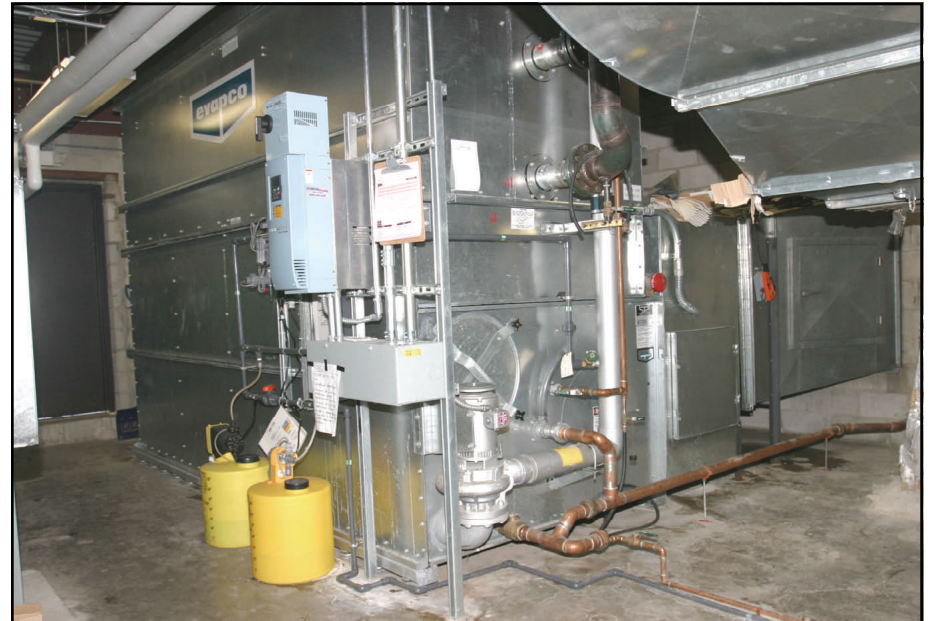
100 Field Point Road Penthouse Mechanicals
